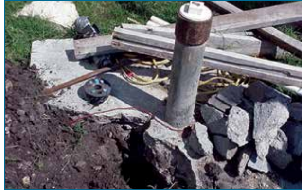
FIGURE 59. The slab around this well is not sufficient to prevent surface contaminants from entering the aquifer. (Source: Plugging Abandoned Water Wells , Bruce Lesikar and Justin Mechell, 2010.)
