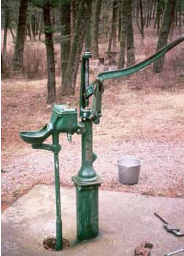
Figure 13—Typical hand pump installation.
