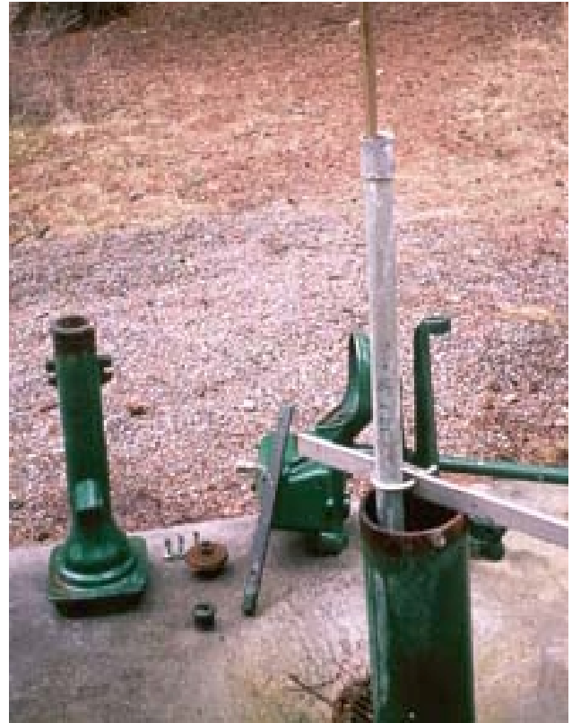
Figure 20—View of clamped drop pipe and pump rod with pump base removed.
