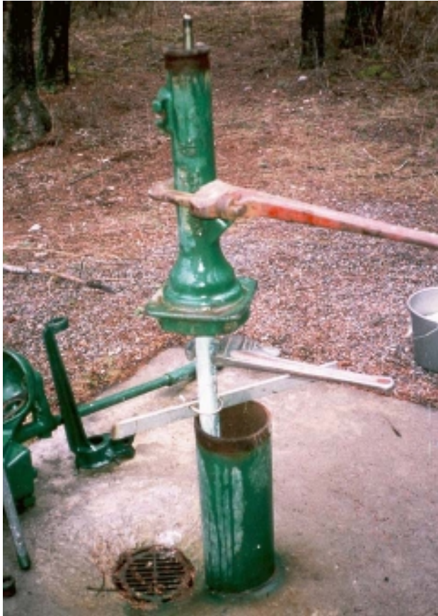
Figure 19—After jack removal, pipe wrenches are applied to the pump base and drop pipe to facilitate rotation of the base to release the drop pipe.
