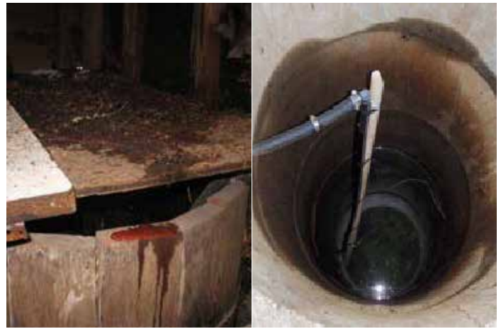
FIGURE 8 Water able to seep into well through the casing
