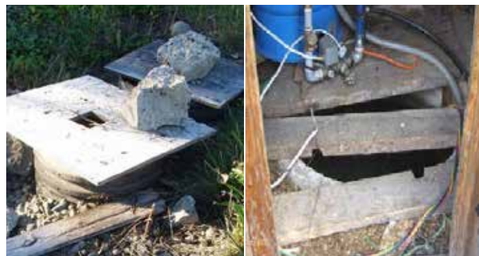
FIGURE 5 Improperly capped wells
