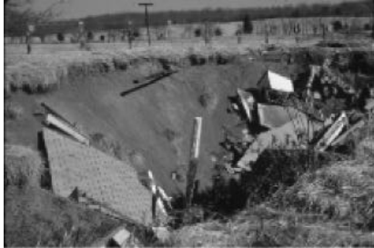
Figure 3. Collapse sinkhole with remains of house, Clarke Co., Virginia.
