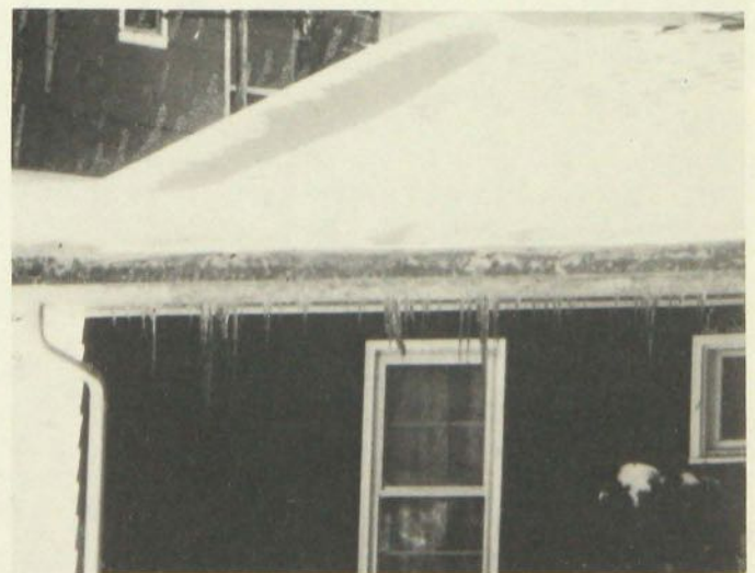
Figure 15. Telescopic lens photo of shrinking and sagging roof-snow on a modern (1962) roof.
