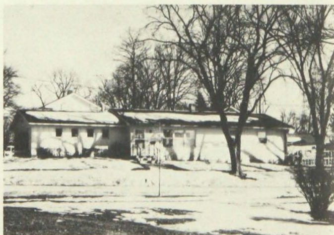
Figure 17. Residual snow pattern on a cold-roof house specifically designed for ice-dam immunity.
