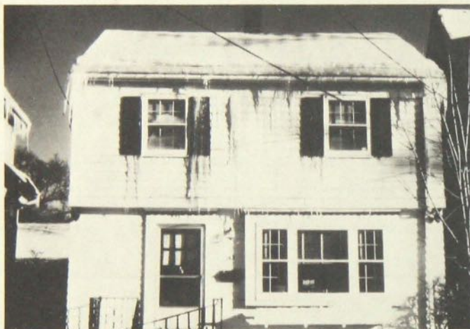
Figure 4. Frozen sidewall leaks emanating from ice-blocked eave.
