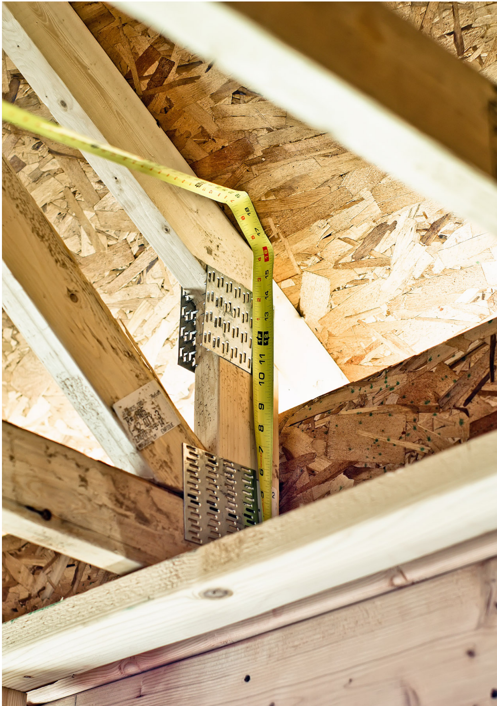
Figure 7. The exterior wall sheathing extends to the top of the raised heel trusses providing structural support for raised heel trusses in high-wind zones (Source: Thrive Home Builders (https://basc.pnnl.gov/library/thrive-home-builders) ).
