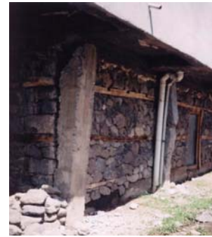
(b) Damaged during Bingöl Earthquake
