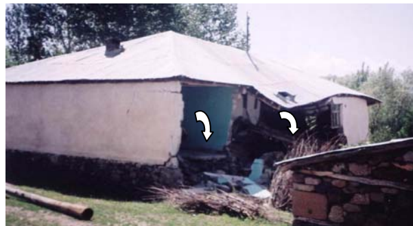
Figure 11 A view of load bearing walls collapsed in the out-of-plane direction during Bingöl Earthquake
