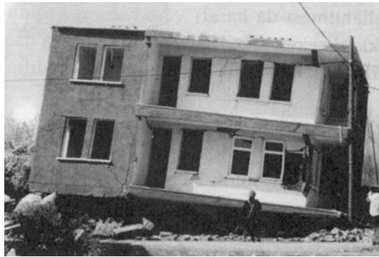
Figure 14 A collapsed building with hollow clay tiles during Sultandağı Earthquake (Ulusay et al, 2002)
