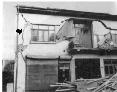
(b) Damaged during Sultandağı Earthquake (Ulusay et al, 2002)
