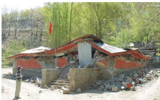
(a) Poor cement mortar in the elementary school building (Emre et al, 2003)
