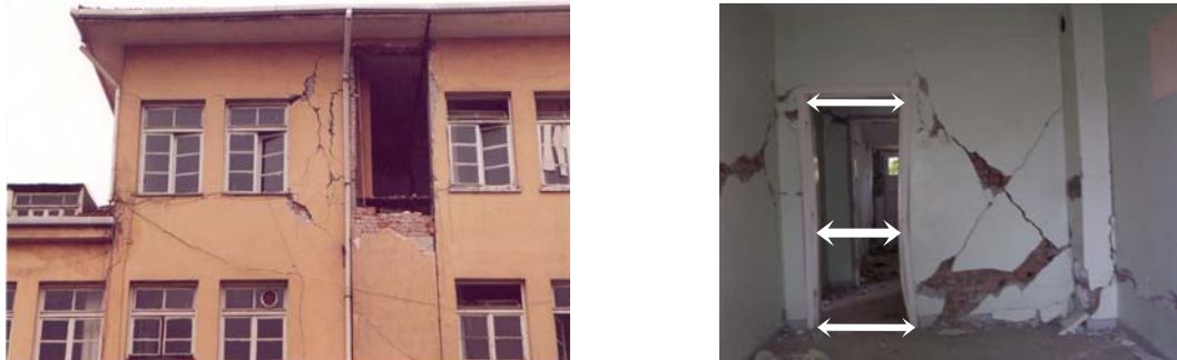
(a) Damage during Kocaeli Earthquake
