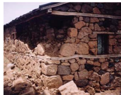
(b) Poor mud mortar
