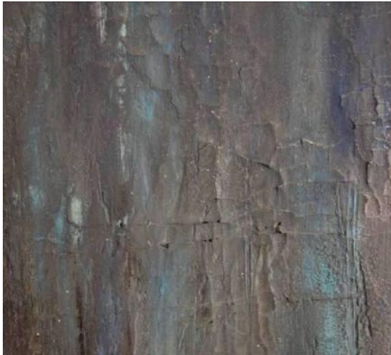
Figure E.06.1 Thick cracking paint in background
