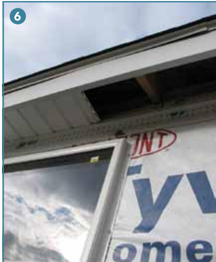
(5) Flames from the window vent out and spread along the vertical obstruction of the soffit. The soffit is made of wood and is not vented, so flames outside of the window will spread to the attic, but not immediately. (Photo by Mike Edelstein, Pittsford Fire Department.)
