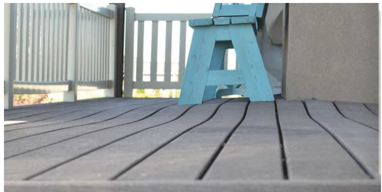
Example above showing the effect on decking when attached to uneven joists/framing.
