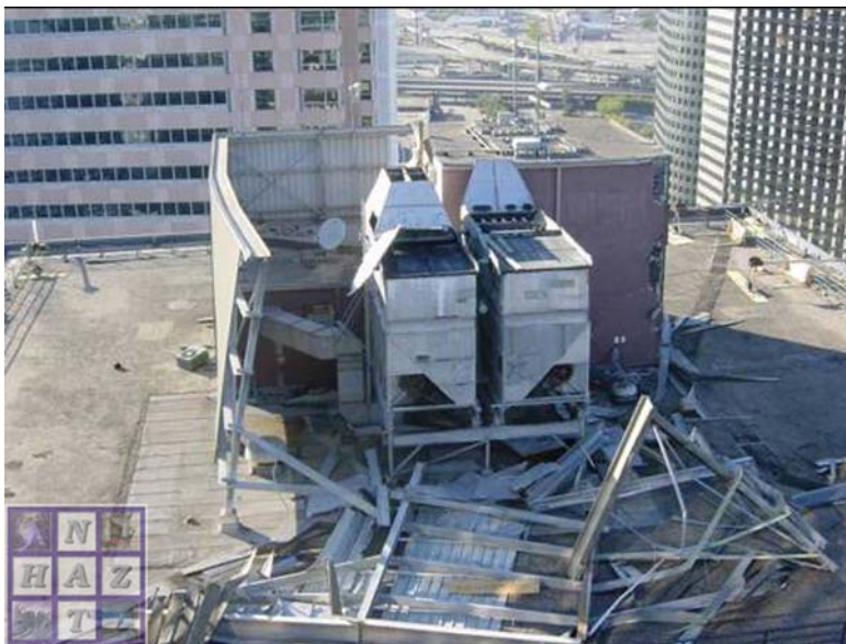
Figure 5 Rooftop penthouse on Amoco Building was nearly destroyed
