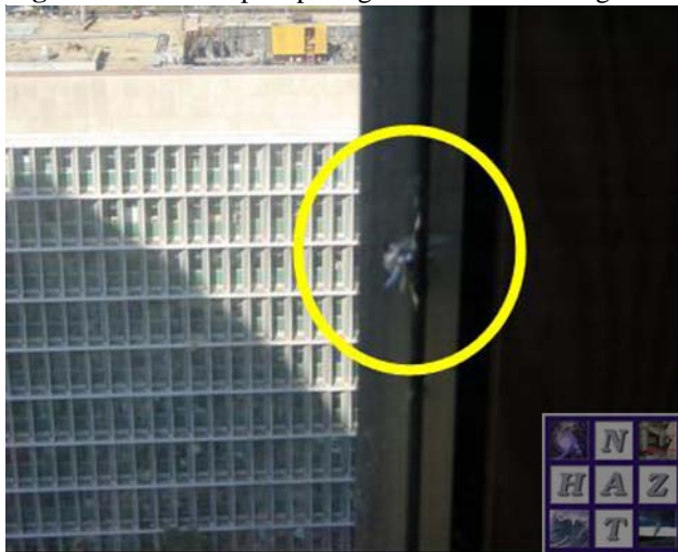
Figure 8 Missile impact pitting on Amoco Building.
