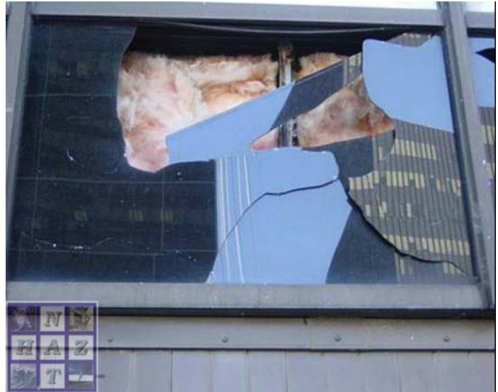
Figure 7 Broken window on north face of Hyatt Regency Hotel, likely caused by missile impact.
