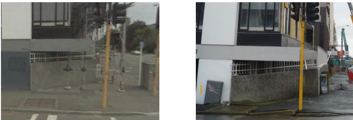
Figure 5.1. Photographs showing corner of structure pre and post 22 February 2011 earthquake event (note height of metal grill above concrete wall, and corresponding damage to pavement)
