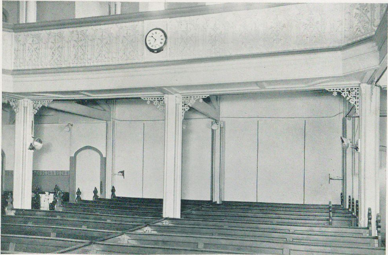
BRUNSWICK STREET METHODIST CHURCH, FITZROY Wall lined with 1" Textured Donnacona over existing wall to correct acoustics.
