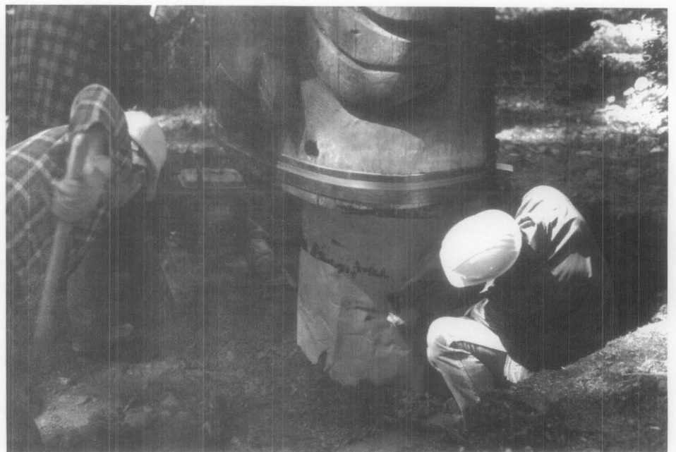
Figure 9. After securing the support post in the ground, a wood preservative in a "bandage" form was attached to the support post before dirt was filled to grade level.
