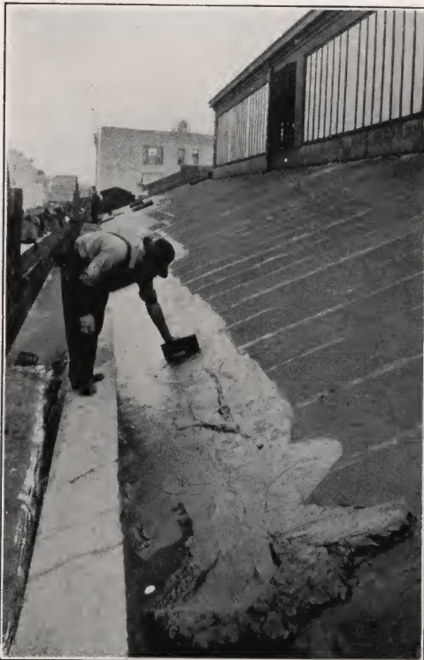
Illustrating application of Plastic Elastigum to S. I. S. Roofing. See page 18
