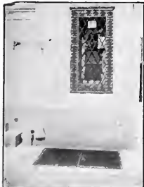
View of Hatch. Sidewalk Doors closed and automatically locked.
