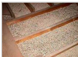
Vermiculite insulation between attic joists; click to view larger version of image
