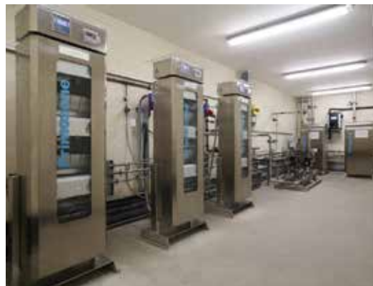
Primozone units installed in series at Yorke WWTP.
