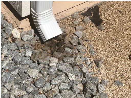
Staining on landscaping (discoloration of aggregate) – Courtesy of Polyglass/S. Wadding
