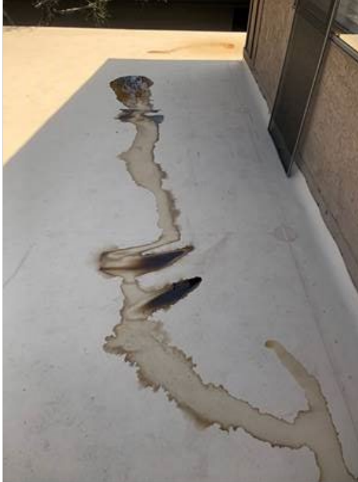
Staining on low-slope roof surface from the upper level.
