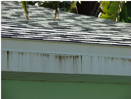
Staining on trim (Courtesy of Owens Corning)
