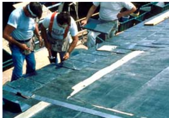
Roofing felt is being installed over the decking; a rubberized membrane is used selectively at the eaves and under some flashing. Photo: NPS files.
