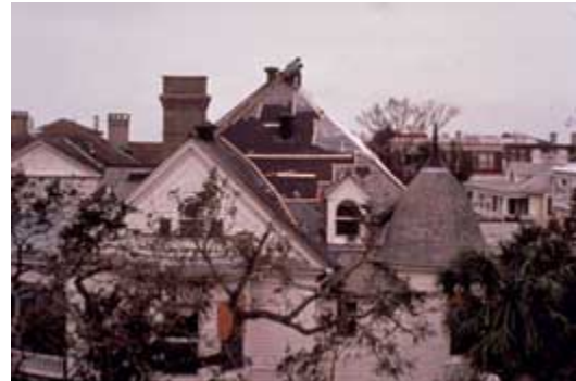
After a hurricane or other natural disaster, it may be necessary to stabilize a roof temporarily until materials can be obtained and a qualified roofing contractor hired. Significant slate roofs should not be stripped off and replaced with asphalt shingles. Photo: NPS files.
