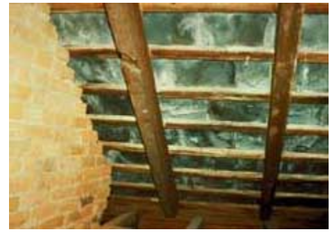
View of these slates laid on open sheathing shows that delamination and flaking are just as bad or worse on the underside of slates as on the exposed surface. This is why most slates cannot be flipped over for reuse. Photo: Jeffrey S. Levine.
