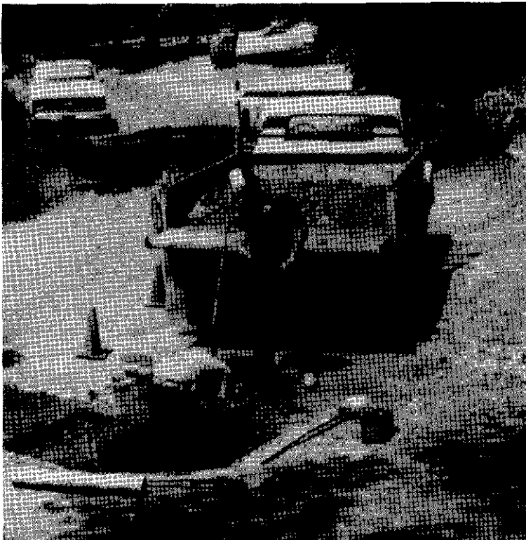
34. Uncovering leaks requires careful excavation to avoid other pipes, other utilities, or both.
