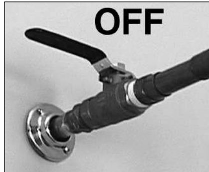
Figure 19 - Cold water supply in off position.
