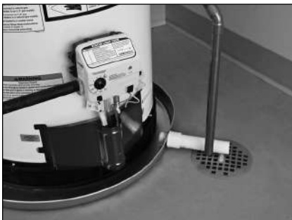
Figure 23 - Metal drain pan piped to drain.
