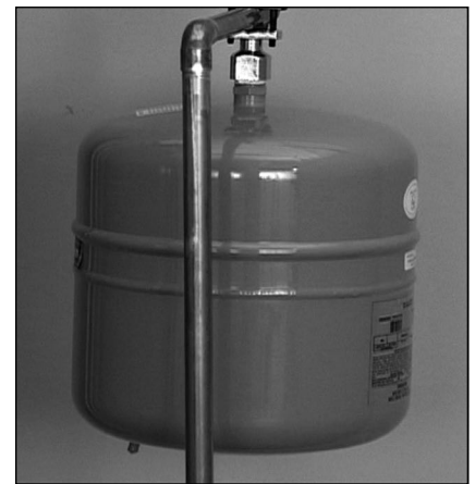
Figure 13 - A Thermal Expansion Tank helps protect the home's plumbing system from pressure spikes.
