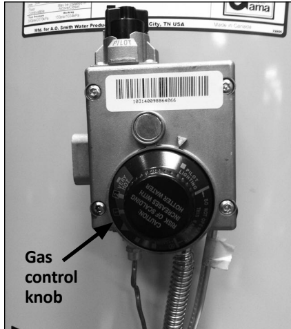
Figure 17 - Turn gas control/temperature knob OFF.
