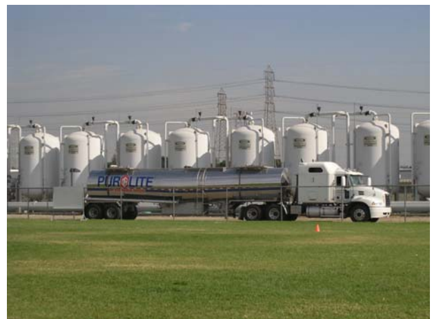
Purolite Bulk Resin Tanker Delivers Perchlorate Selective Resin to a Site in California
