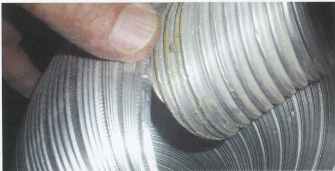
Photo 5. The flex duct from the fan is bad enough, but to air couple it to a bath duct?
