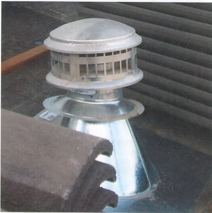
Photo 4. Vent is too close to the roof, too close to the sidewall and too close to the window.
