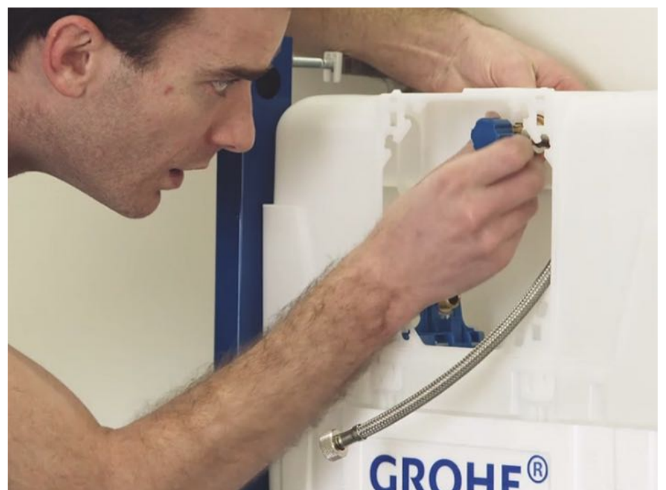
6 - Make sure the isolation valve is closed and open the main water supply. Make sure the isolation valve connection is water-tight.
