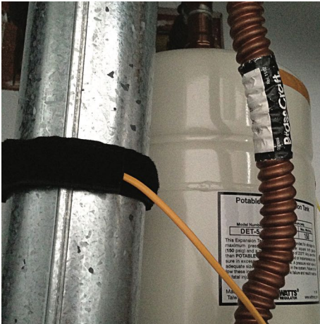
Figure 7. Measuring flue temperature T[\text{flue}] with a Fluke® 80PK-11 strap-on type-K thermocouple provides an accurate indicator of thermostat on/off cycling.
