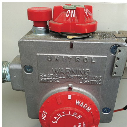
Figure 1. Residential hot-water thermostat set to 120°F temperature range.
