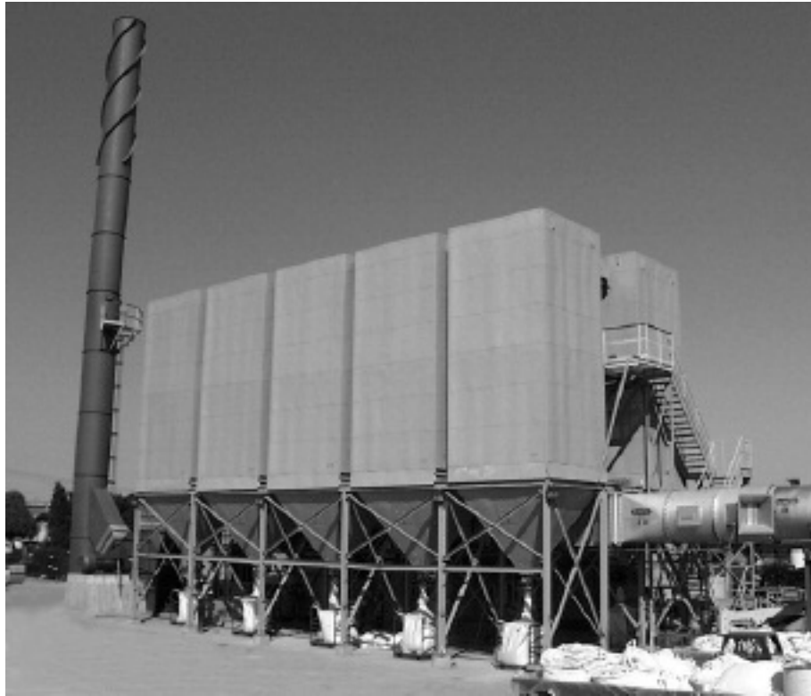
Figure 4—Bag House (Pollution Control Equipment).
