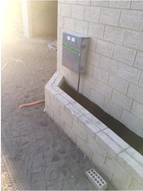
Figure 19: Example of a Gas Meter Box Position Placed On Hold
