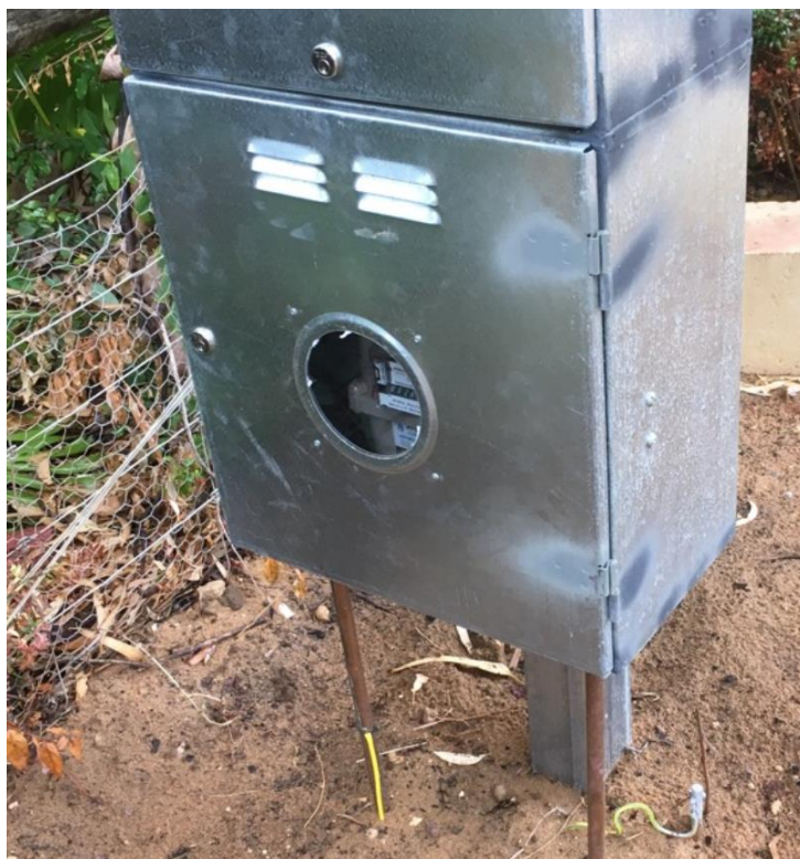
Figure 2: Gas Meter Box Viewing Aperture – Example
