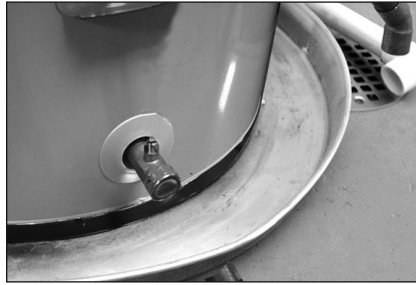
Figure 6 - A suitable drain pan piped to an adequate drain can help protect flooring from leaks and drips.
