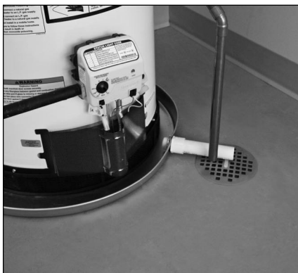
Figure 14 - A metal drain pan piped to an adequate drain can help protect flooring from leaks and drips.
