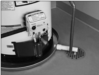
Figure 23 - Metal drain pan piped to drain.
