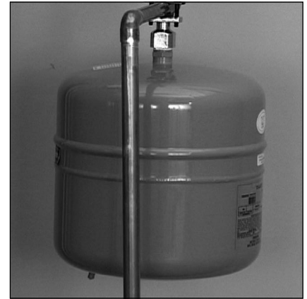
Figure 29 - The Thermal Expansion Tank should be pressurized with air, using a hand pump, to match the home's incoming water pressure.
