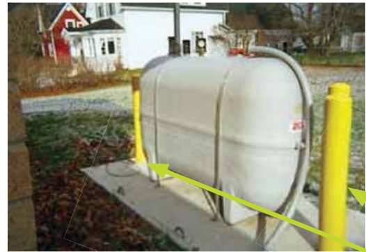
Protect the tank from vehicle impact with posts if no other location is possible.
