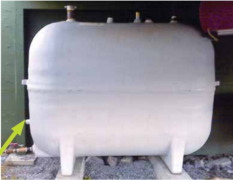
This double-wall fiberglass tank is also fitted with an inspection port to check for leakage.
