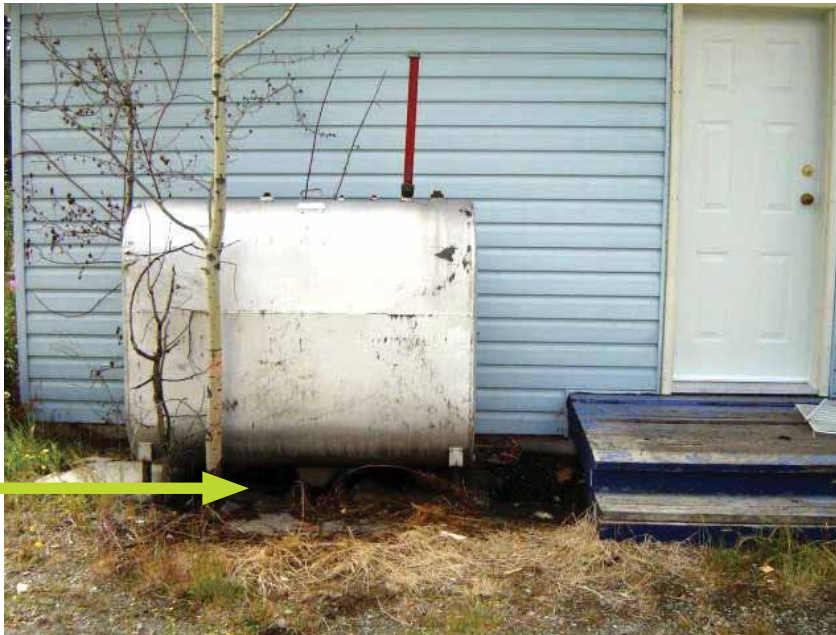
An obvious home-heating oil tank spill. The extent of the spill needs to be determined.
