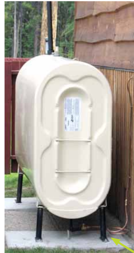
A double-bottom home-heating oil tank on reinforced concrete pads placed on a compacted, granular base.
