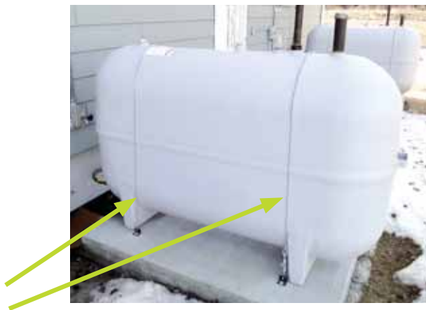
A properly installed fiber glass tank on a solid pad with restraints to keep it from toppling in a seismic event. The restraint system must be engineered or follow certified designs for the local area.
