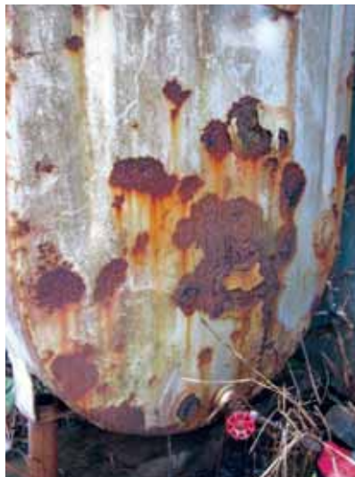
Rust and pitting like this means that this tank is at the end of its life, get it replaced!
