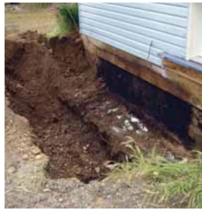
Testing will determine the extent of excavation required to remediate this spill.
