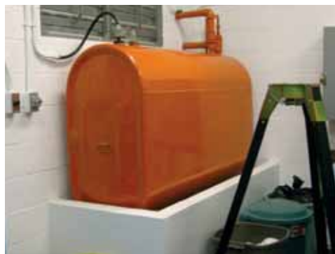
An indoor tank with secondary containment. Notice the fill and vent pipes terminate outdoors.
