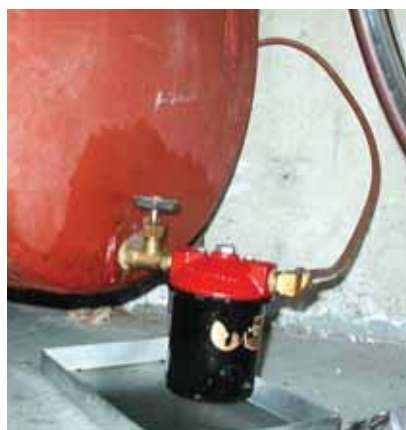
A drip pan under the filter inside a dwelling. The entire tank could have a pan installed beneath it for better protection. Note the appearance of fuel staining on the tank.
