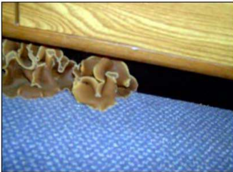
Fruiting bodies of a Peziza sp. in a room with chronic water damage. Peziza sp. is an ascomycete (producing sexual ascospores in a structure called the ascus) and is also known as one of the cup fungi. It is occasionally found on chronically wet or water-damaged wood products (such as plywood subfloor). Peziza can be identified only when the sexual fruiting body is present. In culture, its vegetative state is named Chromelosporium sp. (Image courtesy of Michael Underhill, CIH, CSP of Trident Environmental Services, Inc.)
