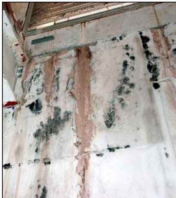
Visible mold growth, including Stachybotrys chartarum , in an outside air-intake plenum in a commercial building. (Image courtesy of Dr. Chin S. Yang of P&K Microbiology Services)
