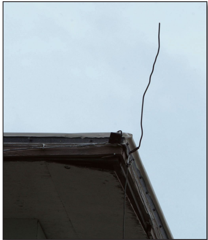
Figure 1a—This improper substitute for an air terminal is made from copper wire.
