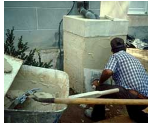
The deteriorated surface of this catch basin is being re-stuccoed. Photo: NPS files.
