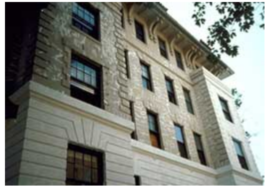
Caulking is not an appropriate method for repairing cracks in historic stucco. Photo: NPS files.
