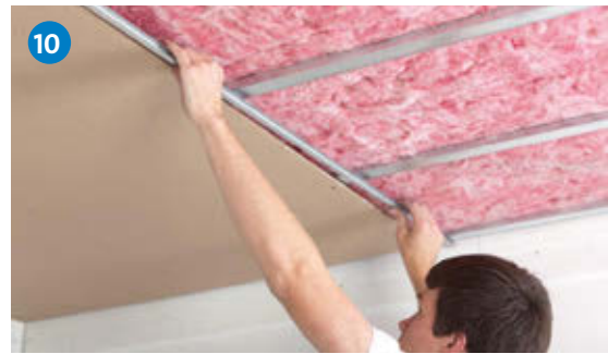
10 After installing the first board, measure and cut M-strip to size and install.
