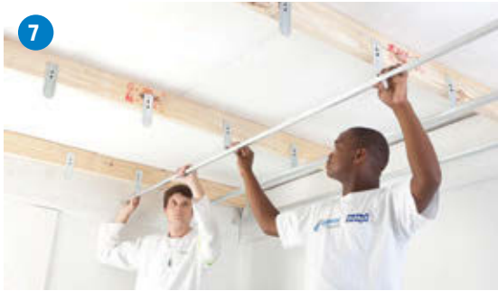
7 Measure and cut steel branding to size and clip onto suspension brackets.
