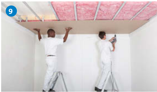
9 Measure and cut RhinoBoard 6.4mm to size. Install the board and fasten using Gyproc RhinoBoard Sharp Point Screws 25mm spaced at 150mm centres.
