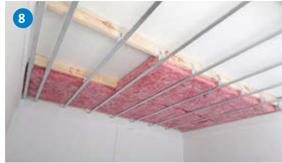
8 After installing the steel branding, install Isovor Aerolite according to SANS 10400-XA for new buildings. (Refer to page 20).
