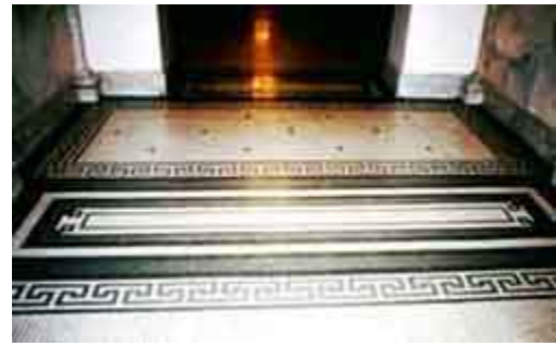
Ceramic mosaic tiles are a practical floor covering in the entryway of this early 20th century school building.
