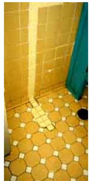
This inappropriate ceramic tile repair is easy to spot. Photo: NPS files.
