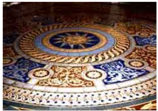
Encaustic floor tiles were decorated with traditional as well as original designs. Over time, the decorations can be worn thin by heavy traffic. Photo: NPS files.
