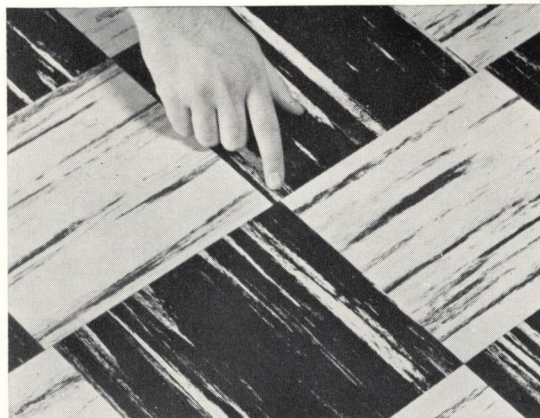
All joints or seam lines should be symmetrical. Uneven lines, such as illustrated above, are more likely to occur in tile installations. Armstrong resilient tiles are die-cut to a perfect square to avoid this condition providing the flooring mechanic squares the room and lays the tiles carefully.
