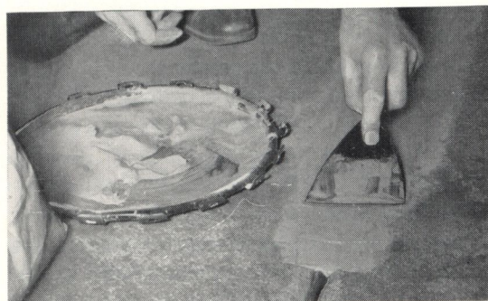
Although resilient flooring adhesives will fill minor cracks and crevices in concrete subfloors, it is best that all conspicuous holes, cracks, and crevices be filled with a reliable cement crack filler before installation is started. It is important that all concrete subfloors be allowed adequate drying time before installing flooring.
