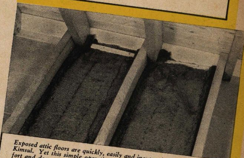
Sloping roofs, usually the most difficult of insulating jobs, are generally an easy "one-man" job with Kimsul! Laths nailed across framing members provide temporary support.
