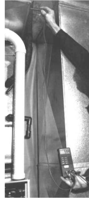
FIGURE 49 TEMPERATURE RISE MEASUREMENT
