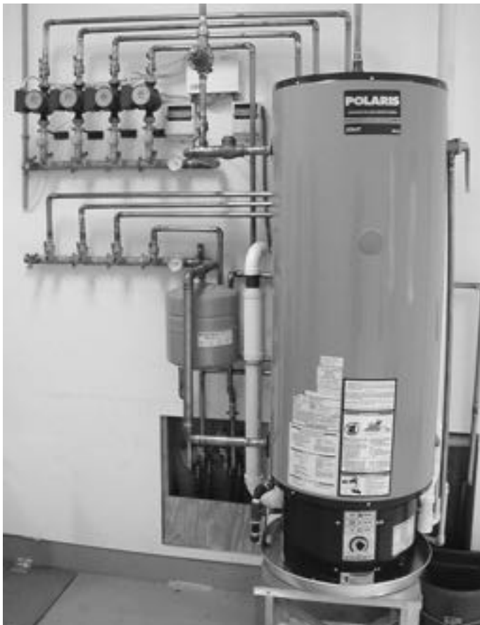
Over a mile of 7/8" PEX was installed in the floor of this state of the art dog kennel in northern Vermont. A 50 gallon, 199,000 BTU/hr., Polaris water/space heater powers a four zone open system and provides the kennel's domestic hot water.....all at 95% efficiency!
