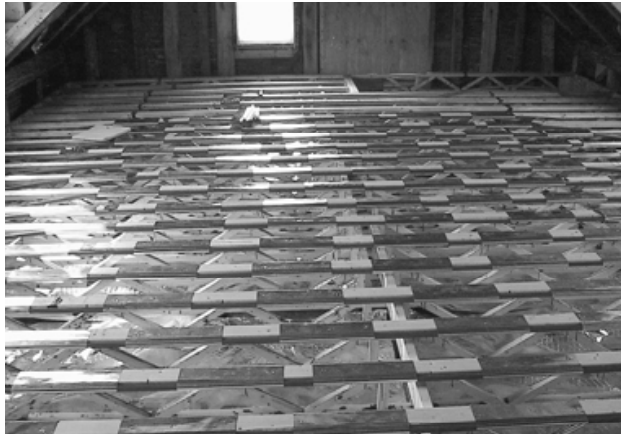
These 9" trusses are insulated from the floor below with 6" of fiberglass that has been covered with a layer of radiant reflective barrier. This guarantees that the radiant heat will flow up into the newly remodeled master bedroom.
