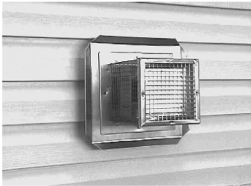
Typical Standard Vent Terminal Installation.
