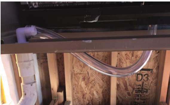
Figure 34: Inside of unit at return-air duct flange, showing sealed condensate tube opening
