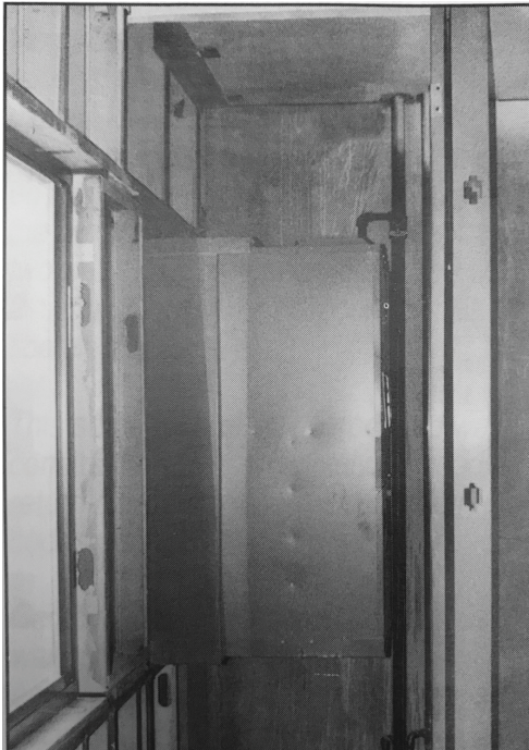
Figure: 29: Wall sleeve fastened to steel 2” x 4” studs with screws fasteners shot through sides of wall sleeve.
