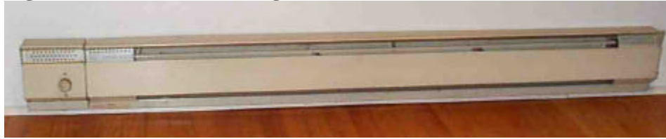
Figure 2: Baseboard Heating Unit
