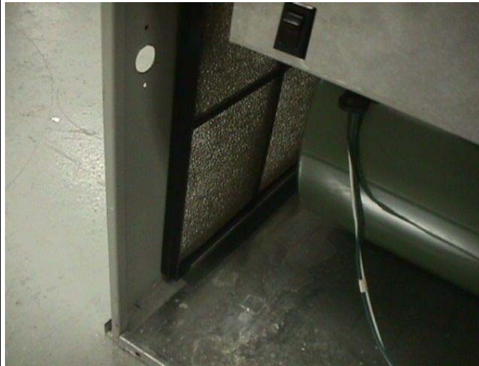
Figure 43: Air filter Maintenance.
