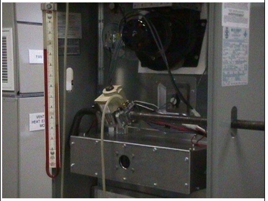
Figure 33: Manometer measuring gas inlet pressure.
