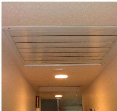
Figure 4-38: Whole-House Fan With Barometric Damper
