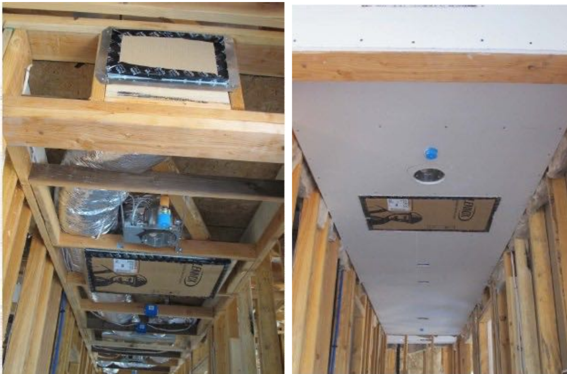
Figure 4-11: Ducts Routed Through a Dropped Ceiling
