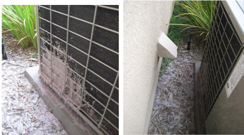
Figure 4-2: Noncompliant Condensing Unit Clearance From Dryer Vents
