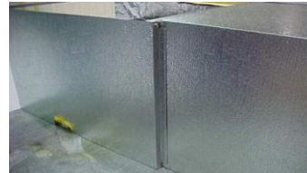
Back of HD coil (left) connected to a blower (right).
