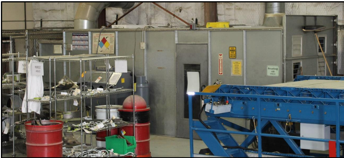
Figure 2-13. Ventilated Walk-in Booth Where Brakes Pads Are Replaced Photograph courtesy of NASA
